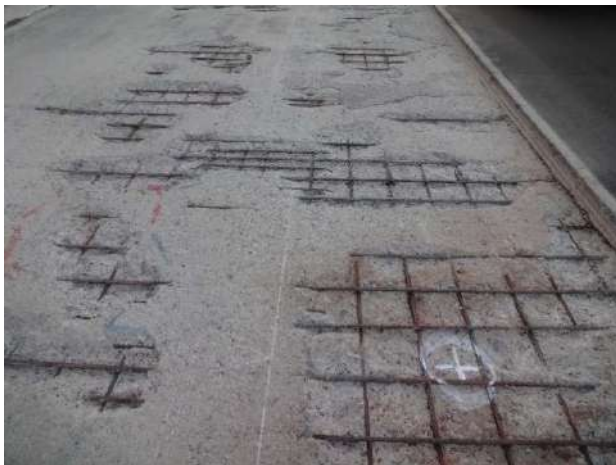
Photo-1 Deterioration of the upper surface of the slab
