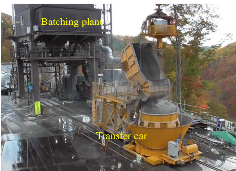
(c) Concrete conveyance facility
